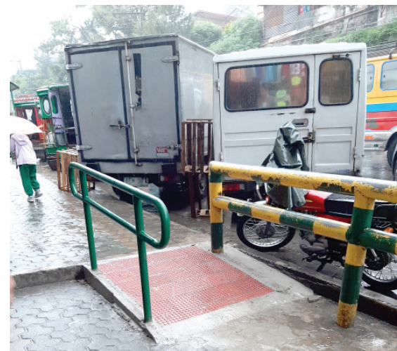
RAMP OF COMFORT – Persons with disabilities and wheelchair-bound individuals can now conveniently access the city market through ramps like this installed along 1st Kayang St. by the DPWH as part of the aim to make roads and facilities accessible to PWDs under Batas Pambansa Bilang 344. – Aileen P. Refuerzo photo.
