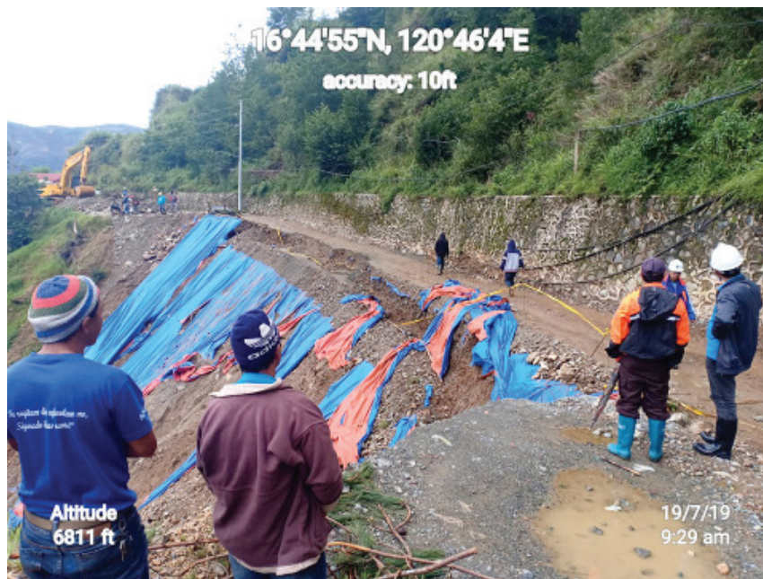
ROAD CLOSED: The Mogao Section of Bakun, Benguet along Acop-Kapangan-Kibungan-Bakun National Road (Gov. Bado Dangwa Road) is closed due to road slip./Bakun-MDRRM
